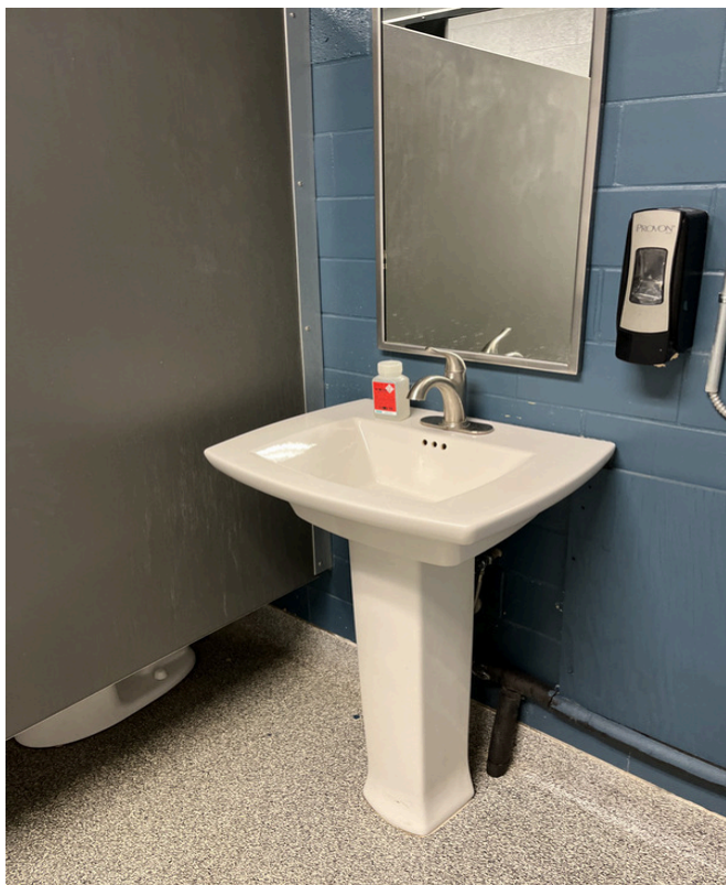
3/12/2024 - 5801-58 - Midway R-1 - Women's Restroom Across From Principal's Office - Closest To Door
