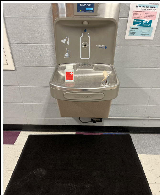
3/12/2024 - 5801-10 - Midway R-1 - Outside Men's Restroom Across From Cafeteria
