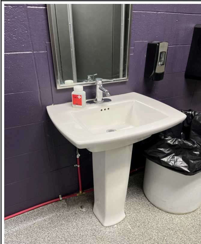
3/12/2024 - 5801-8 - Midway R-1 - Men's Restroom Across From Cafeteria - Furthest From Door
