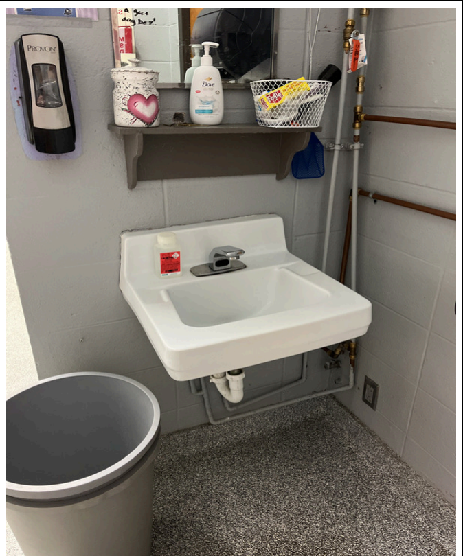
3/12/2024 - 5801-17 - Midway R-1 - Kitchen - West Handwashing Station
