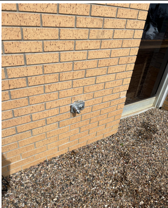
3/12/2024 - 5801-88 - Midway R-1 - North Exterior Outside Room 202 - Out Of Order
