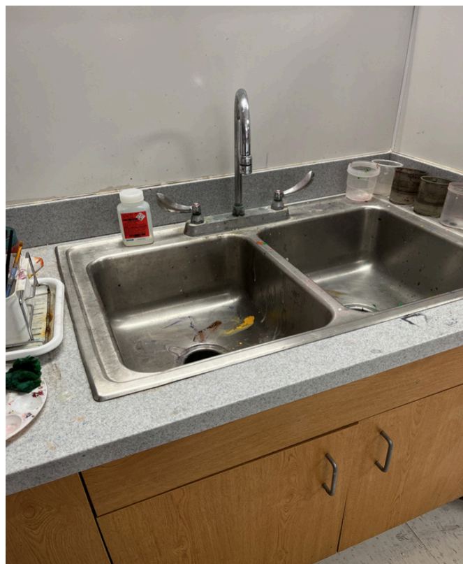
3/12/2024 - 5801-24 - Midway R-1 - Room 210 -South Sink
