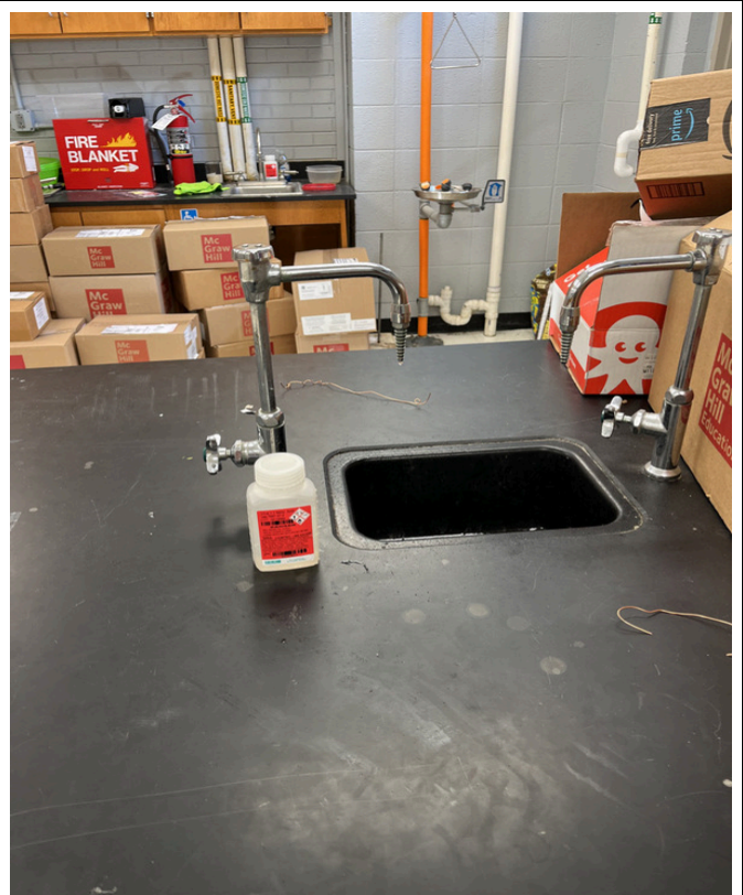
3/12/2024 - 5801-72 - Midway R-1 - Room 109 - South - Furthest From Door - Left
