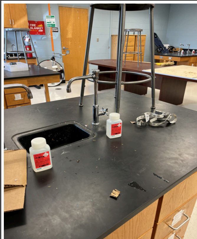
3/12/2024 - 5801-30 - Midway R-1 - Room 202 - South Side - Middle Row - Right Faucet
