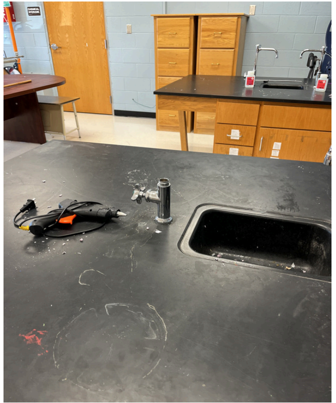
3/12/2024 - 5801-35 - Midway R-1 - Room 202 - North Side - Middle Row - Left Faucet - Out Of Order
