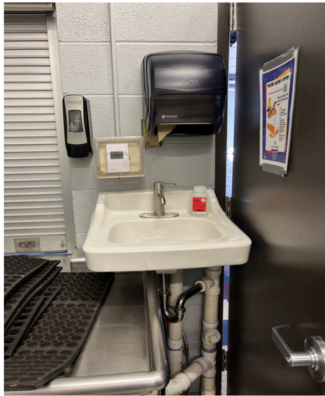
3/12/2024 - 5801-22 - Midway R-1 - Kitchen - North - Handwashing Station
