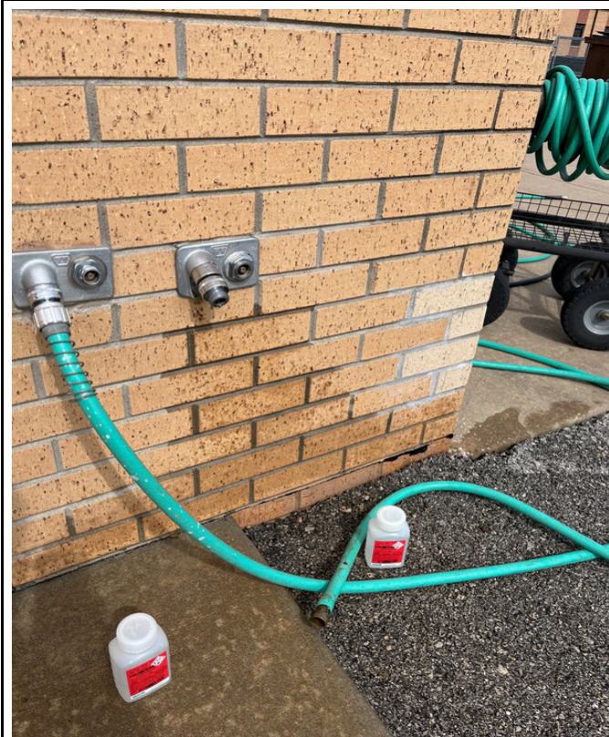
3/12/2024 - 5801-89 - Midway R-1 - North Exterior Outside Room 210 - Right
